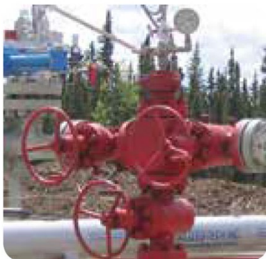
Wellhead Gate Valve
